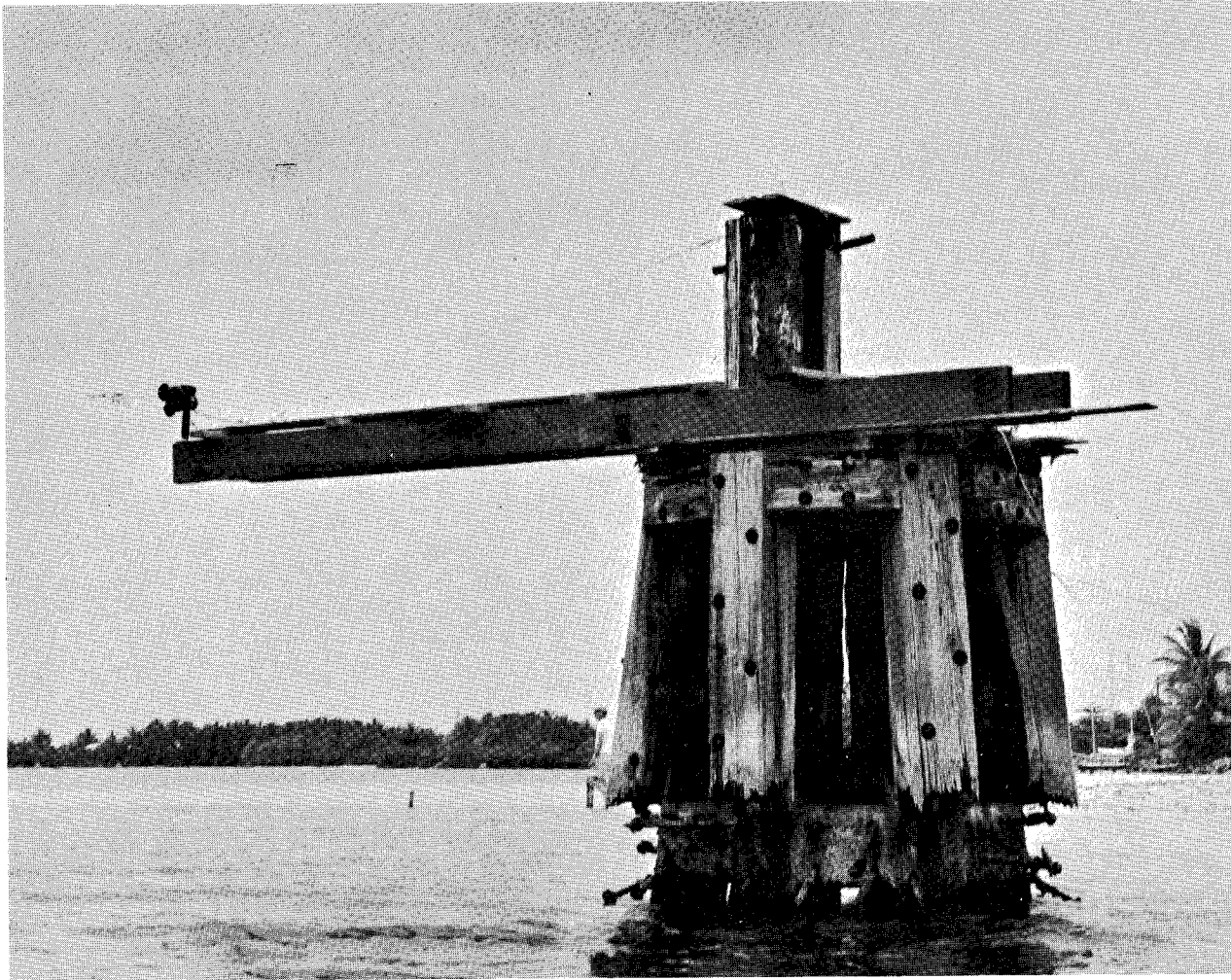
Fig. 11 Piling in Palmyra lagoon serving as radiometer site. The net infrared radiometer is suspended over the lagoon on the extreme left. (NCAR photo)
