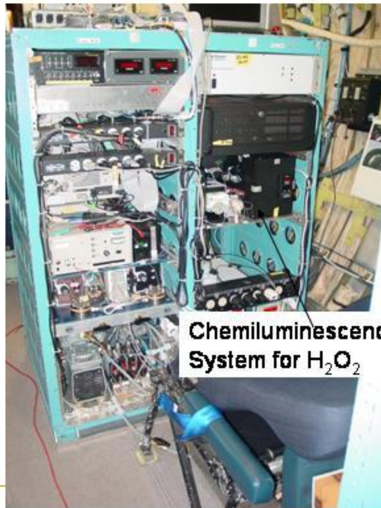
Instrument Rack Aft Facing View
